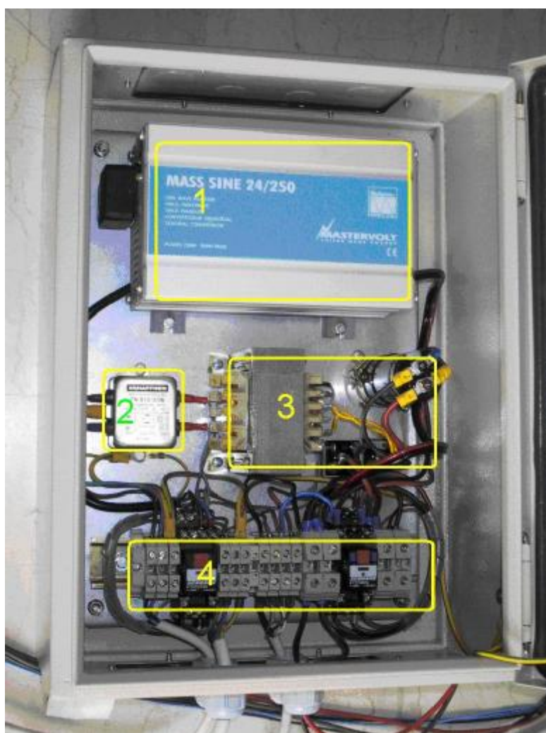
Power Supply Enclosure
